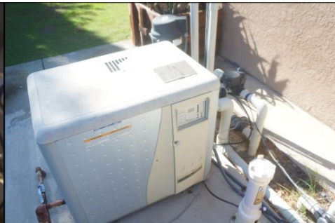
SPA Heating System
