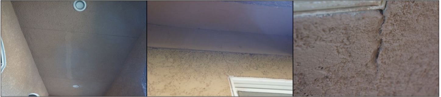
EXTERIOR WALLS Stucco/EIFS Cracking EXTERIOR WALLS Stucco/EIFS Cracking EXTERIOR WALLS Stucco/EIFS Cracking
