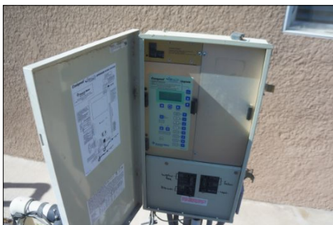
SPA Control Systems
