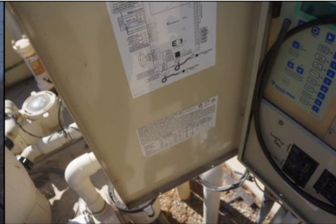
SPA Control Systems
