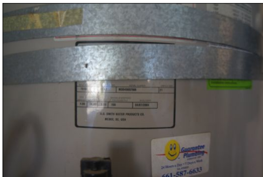
WATER HEATER Water Heater Data Plate Information
