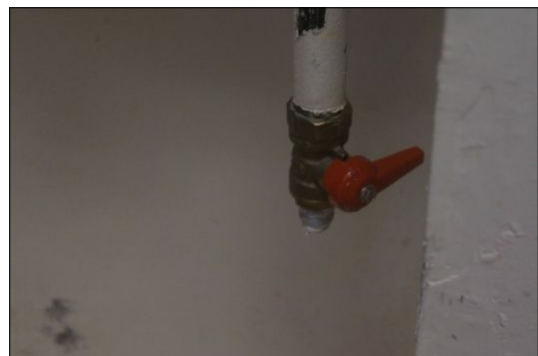
LAUNDRY Plumbing Connections
