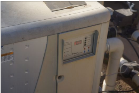
SPA Heating System
