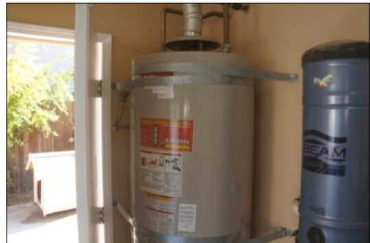
WATER HEATER General Condition
