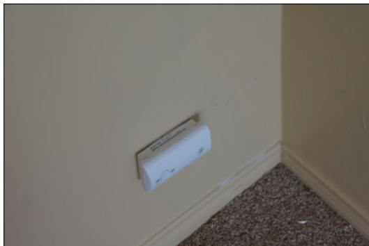
MASTER BEDROOM Smoke/CO Detectors
