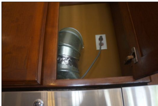
KITCHEN Range Hood
