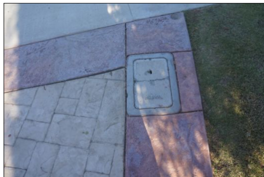
PLUMBING Water meter
