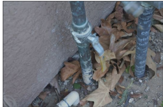
PLUMBING Main Water Pipe/Shut-off
