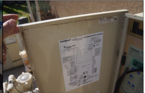
SPA Control Systems
