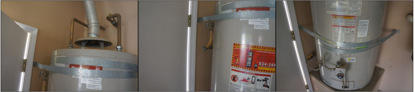
WATER HEATER General Condition
