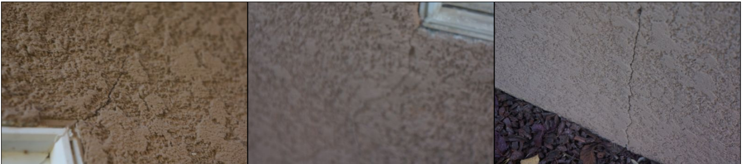
EXTERIOR WALLS Stucco/EIFS Cracking EXTERIOR WALLS Stucco/EIFS Cracking EXTERIOR WALLS Stucco/EIFS Cracking
