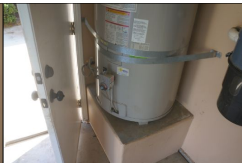
WATER HEATER General Condition
