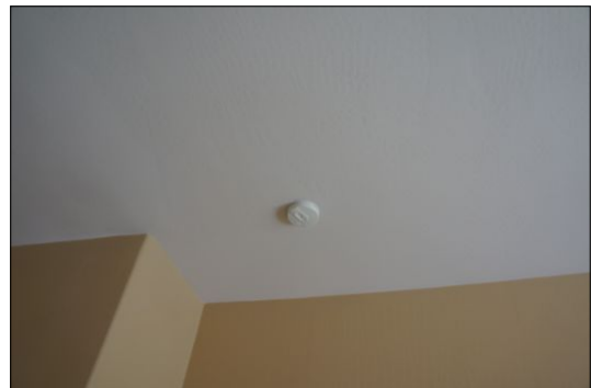
MASTER BEDROOM Smoke/CO Detectors
