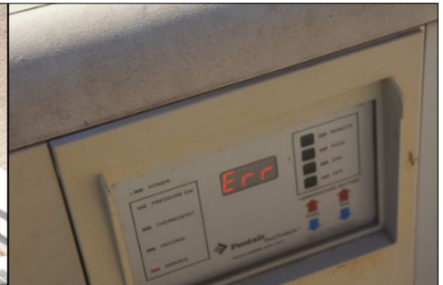
SPA Heating System
