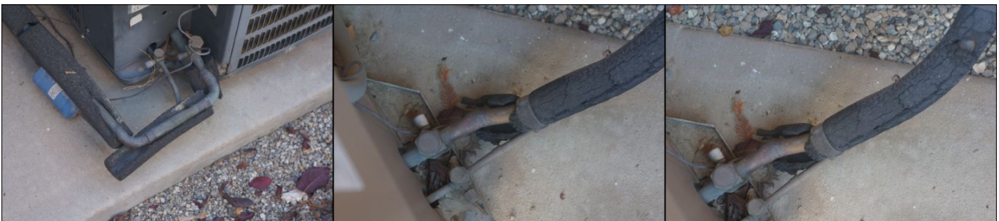
CENTRAL AIR CONDITIONING AC Refrigerant Lines
