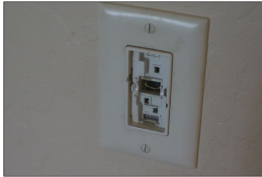
ELECTRICAL Lighting Fixtures
