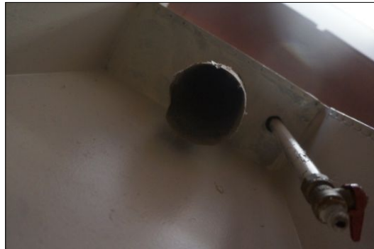
LAUNDRY Dryer Venting
