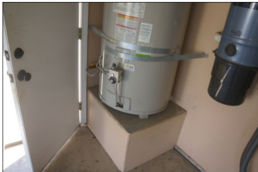
WATER HEATER General Condition
