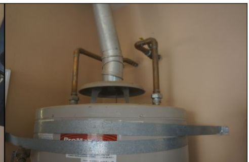
WATER HEATER General Condition
