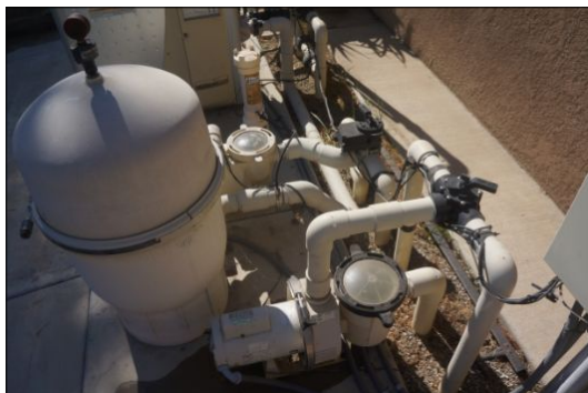
POOL Plumbing System
