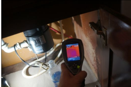
KITCHEN Undersink Conditions
