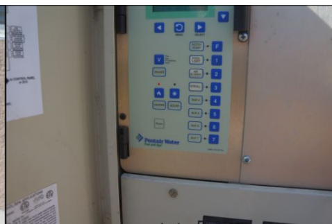
SPA Control Systems
