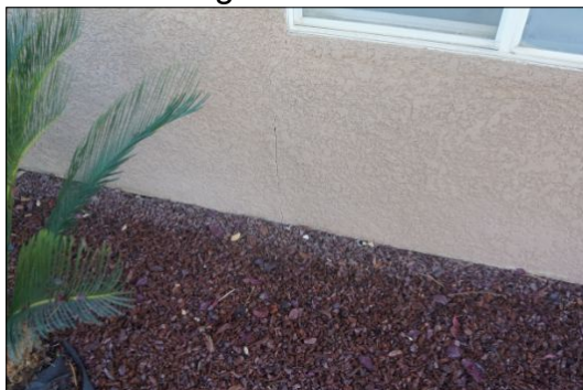
EXTERIOR WALLS Stucco/EIFS Cracking
