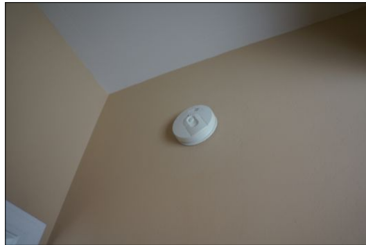
GENERAL INTERIOR Smoke/CO Detectors
