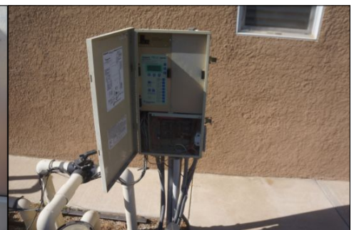
SPA Control Systems
