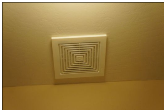
MASTER BATHROOM Bathroom Ventilation
