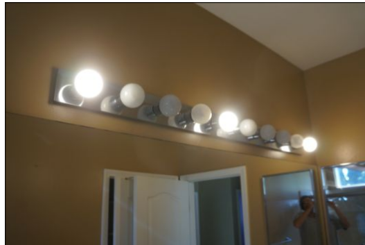
BATHROOM 3 Light Fixtures
