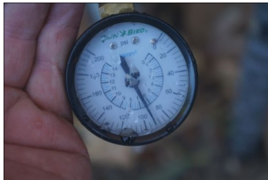
PLUMBING Water Pressure
