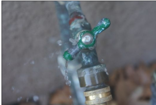
PLUMBING Exterior Faucets
