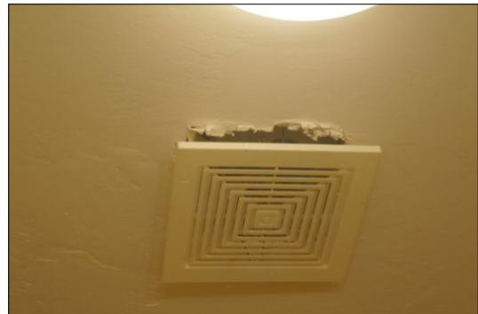
BATHROOM 2 Bathroom Ventilation
