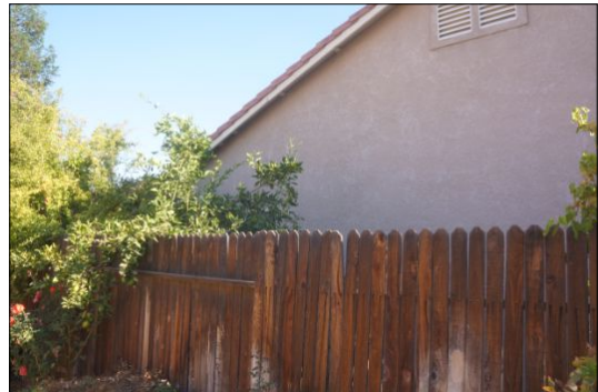
GROUNDS Fence Condition
