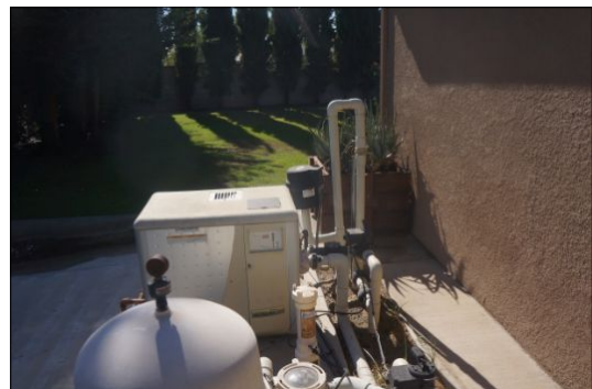
POOL Plumbing System
