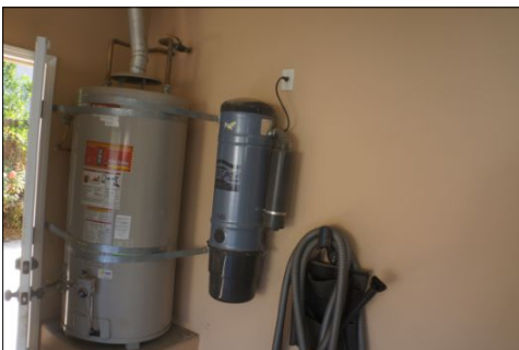
WATER HEATER General Condition
